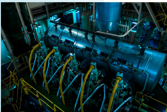
Machinery Status Alerts
